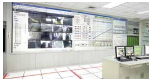
Digital central-monitoring systems
