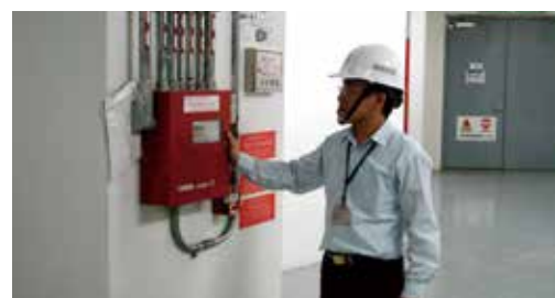
Daily maintenance of the firefighting equipment
